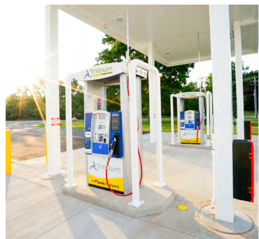
Compressed Natural Gas Station Junction Ave, San Jose
