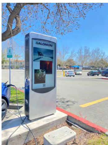
Electric Station West Park Plaza, San Jose
