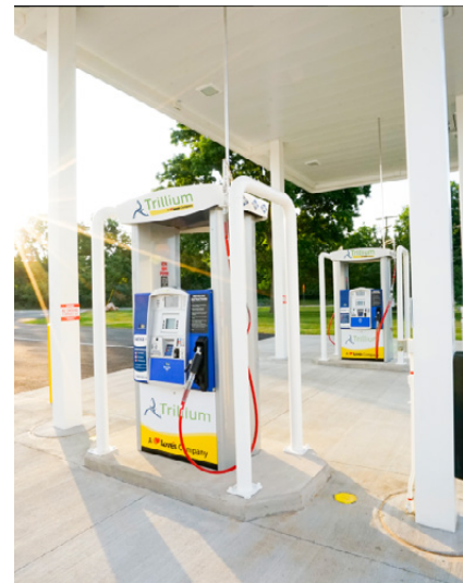
Compressed Natural Gas Station Junction Ave, San Jose
