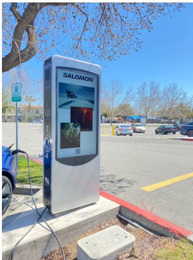
Electric Station West Park Plaza, San Jose
