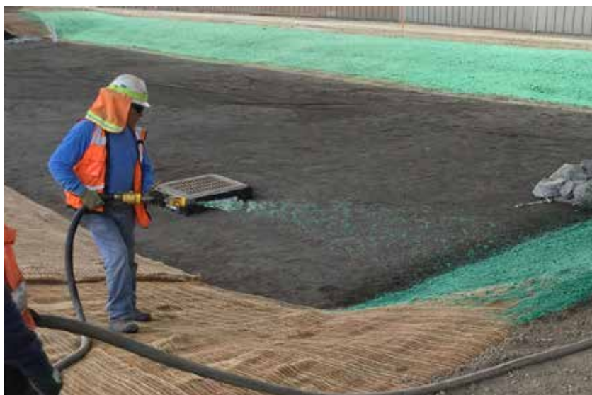
Figure 7: Bioretention basin is adequately protected from construction run-on using temporary hydromulch and erosion control blanket.
