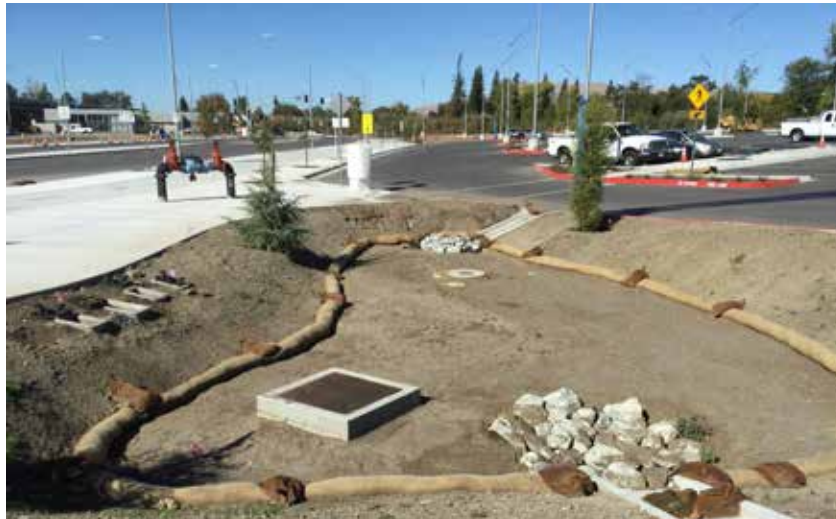
Figure 6: Bioretention basin is inadequately protected with only fiber rolls. Note the accumulated sediment filling the rock riprap and discoloring the soil media on the left half of the basin.
