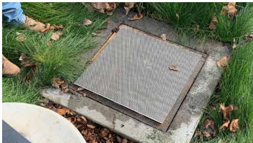
Figure 19: 5mm Trash Screen on Bioretention Basin
