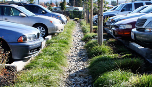
Bioswale and Planting with Trees
