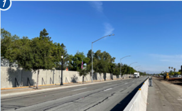
Capitol Expressway is widened in some areas to allow room in the median. This space is needed to facilitate the movement of heavy equipment and build the guideway. Temporary noise walls were installed parallel to construction.
