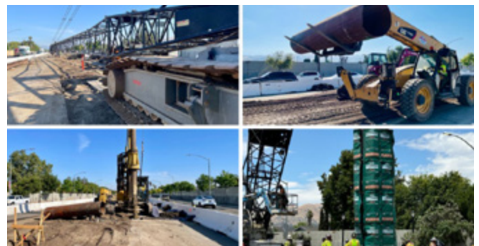
Construction activities began on May 2024 along the 2.4-mile construction zone on Capitol Expressway. (Photo: VTA/LP)
