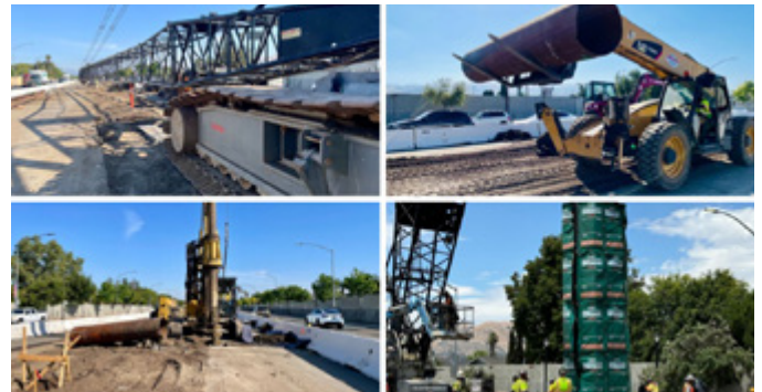
Construction activities began on May 2024 along the 2.4-mile construction zone on Capitol Expressway. (Photo: VTA/LP)
