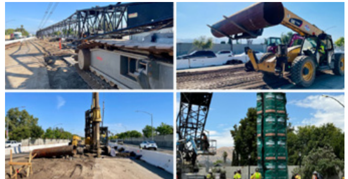
Construction activities began on May 2024 along the 2.4-mile construction zone on Capitol Expressway. (Photo: VTA/LP)
