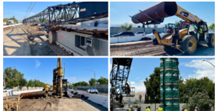
Construction activities began on May 2024 along the 2.4-mile construction zone on Capitol Expressway. (Photo: VTA/LP)
