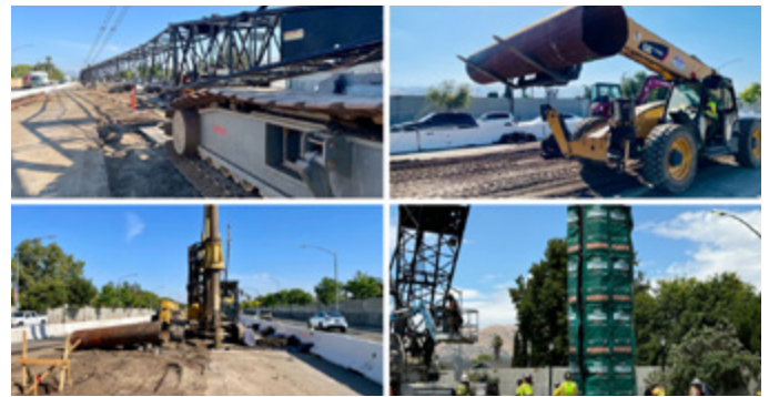
Construction activities began on May 2024 along the 2.4-mile construction zone on Capitol Expressway. (Photo: VTA/LP)
