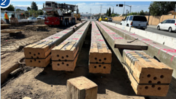
Piles are driven to 80 feet deep. These piles will support the columns.
