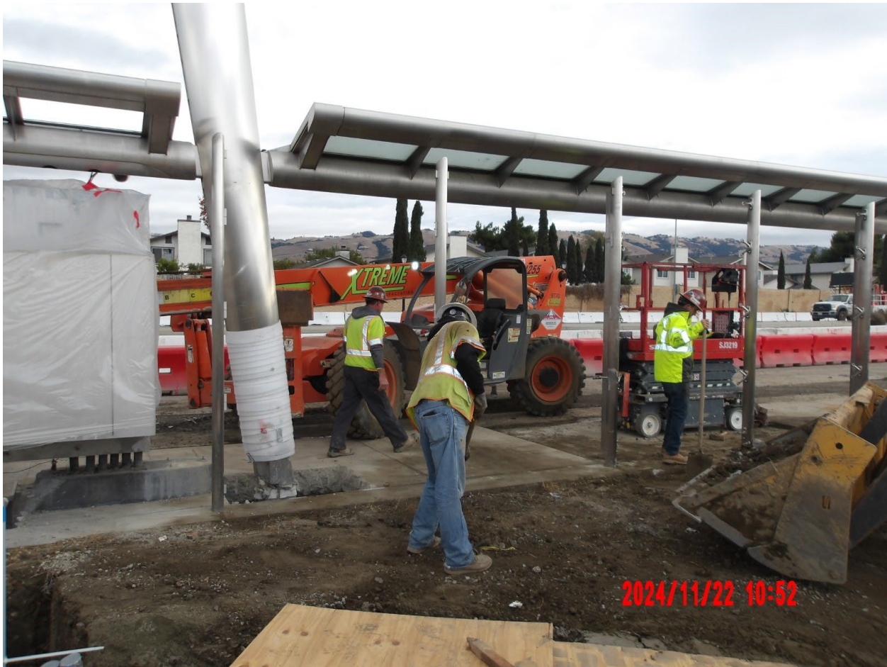
Workers continue to dismantle BRT station shelter to be relocated after roadway widening. [Photo by MCM Construction/VIS]
