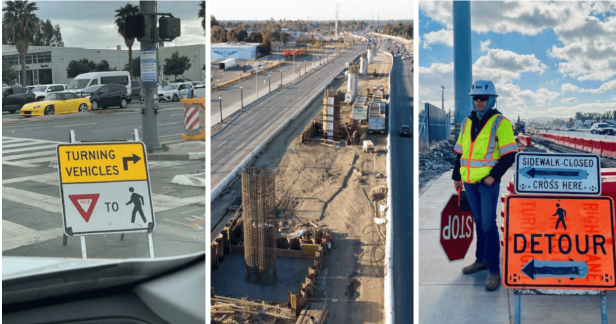
(Left to Right) – A) “Yield to Pedestrians,” and other traffic and construction signs are noticeable throughout the construction zone. B) Construction columns are being built along Capitol Expressway. C) A flagger assists pedestrians and bike riders on Capitol Expressway, close to the Tully Road intersection. [Photos by VTA/EBRC SF&LFP].
