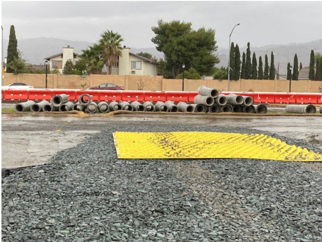
Gravel and other protections are in place to reduce mud tracking by vehicles from rain. [Photo: MCM/VS]
