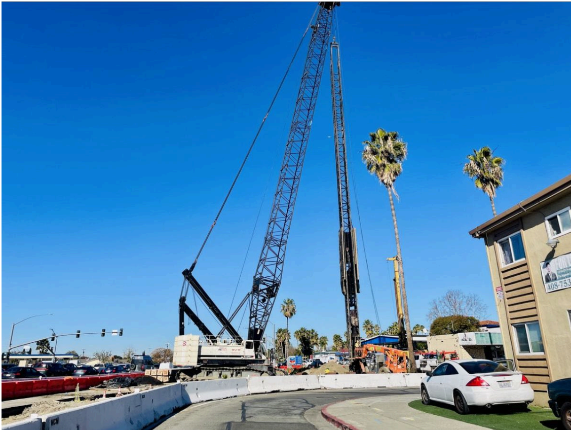
(East San Jose) – Construction crews paved certain areas on South Capitol Ave., westside of Capitol Expressway, ahead of the expressway’s expansion to build the aerial guideway of the EBRC. [Photo VTA/EBRC LFP].
