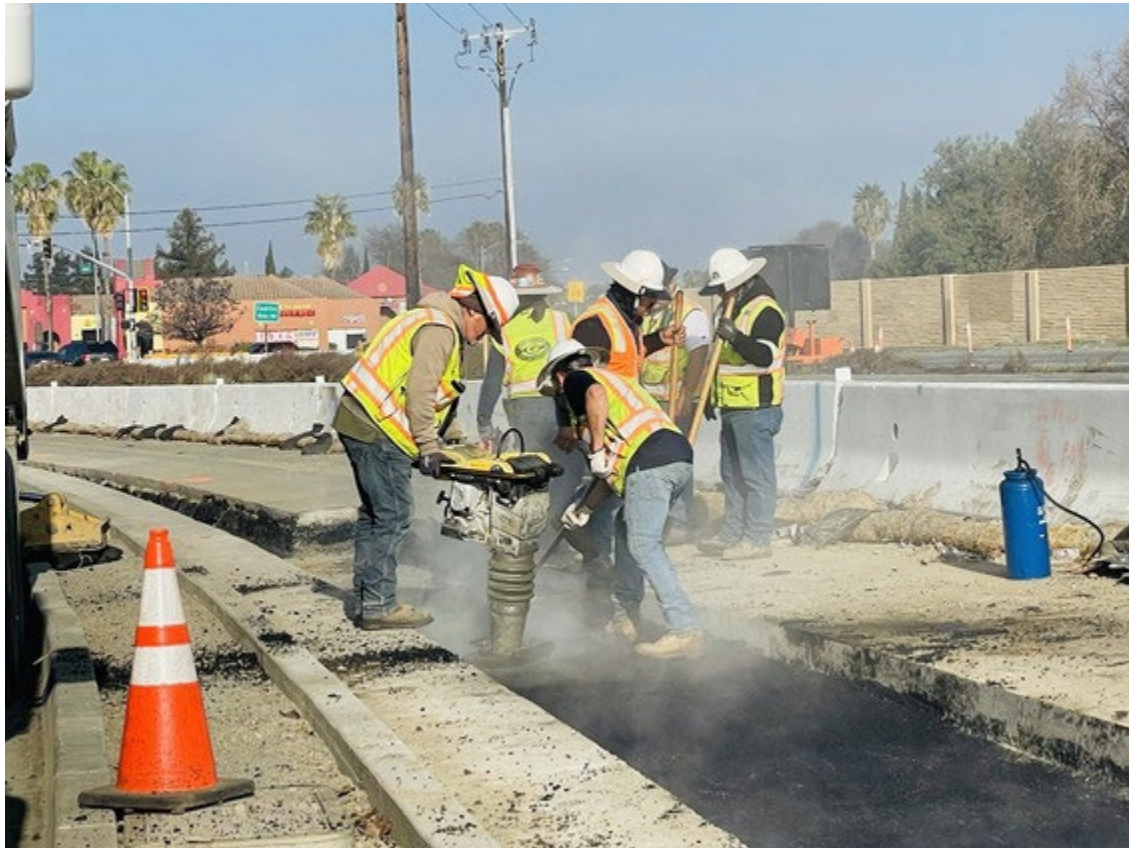
Crews placing asphalt on S. Capitol Avenue near Excalibur Drive. [Photo VTA/EBRC LFP].
