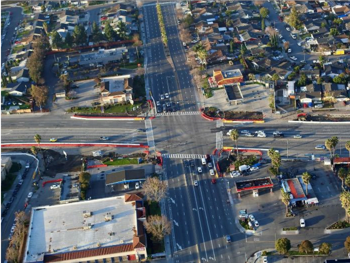
Aerial view of Story Road Intersection under construction with pedestrian paths next to orange barriers [Photo by VTA/EBRC].
