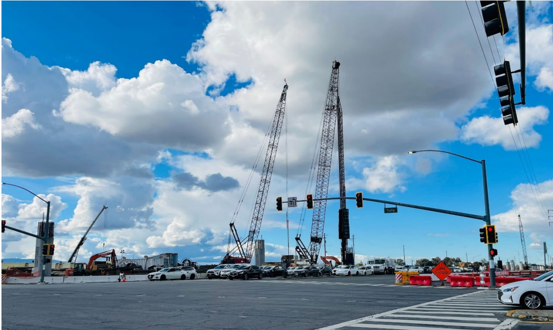
Cranes stand on the northwest corner of Capitol Expressway and Tully Road for sheet and pile driving to build the foundation/ columns that will support the guideway transition from the median to the west side of Capitol Expressway. [Photo VTA/EBRC LFP].
