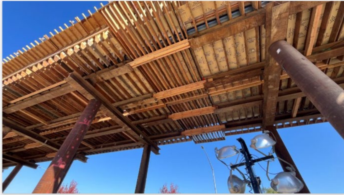
Temporary support system for the new VTA Guideway on Capitol Expressway. [Photo by Bill Faoro/MCM Construction].
