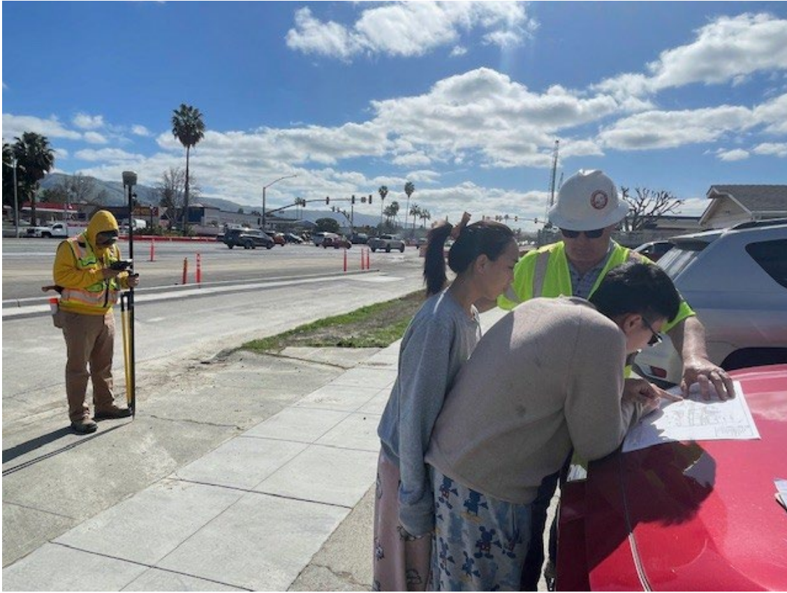
Resident Engineer Scott Hensler explains to homeowners the upcoming construction activities in front of their home while a surveyor ensures the accurate layout for the upcoming roadway, sidewalk, and driveway activities. [Photo: VTA/EBRC LFP].
